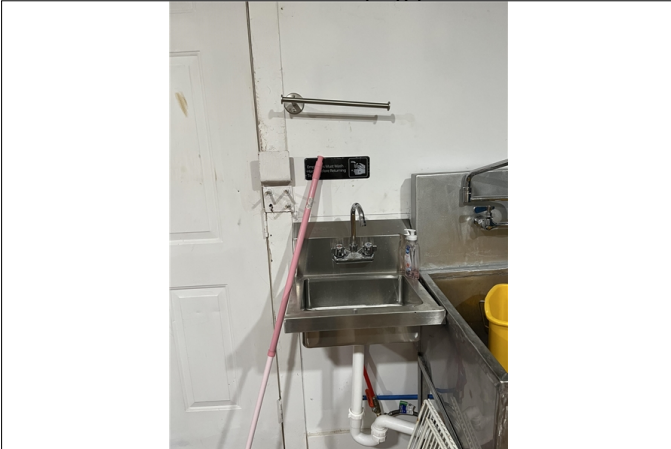
back sink no drying provisions
