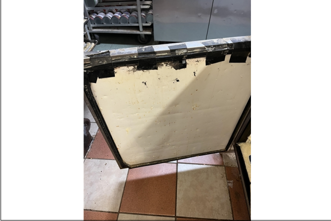
door poor repair
