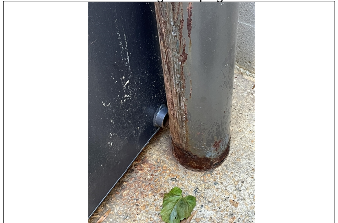
missing drain plug #2
