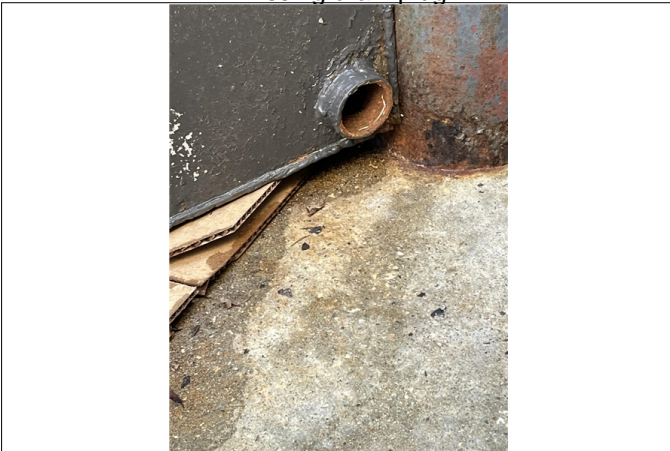
missing drain plug #1
